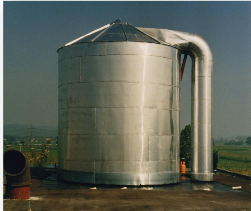
Installation inside building vs. above roof
